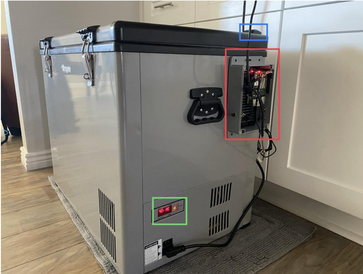
Figure 2: Active cooler unit. Red: Able Temp Cloud connected monitoring device. Blue: GPS receiver. Green: LCD display for cooler.
